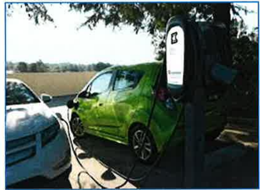
Electric Car Recharging
