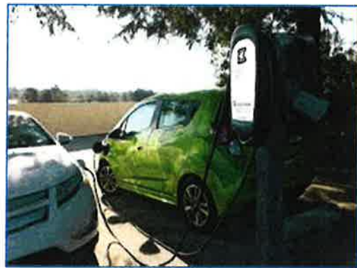
Electric Car Recharging
